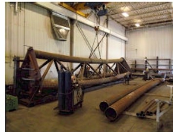
The 2 nd and 3 rd sections of 6 trusses which form the 240' span arch, being prepared by DEPCO. Each section weighs between 6 and 9 tons and will be bolted together in the field. The entire arch will then sit on four 6" diameter shear pins when erected.
