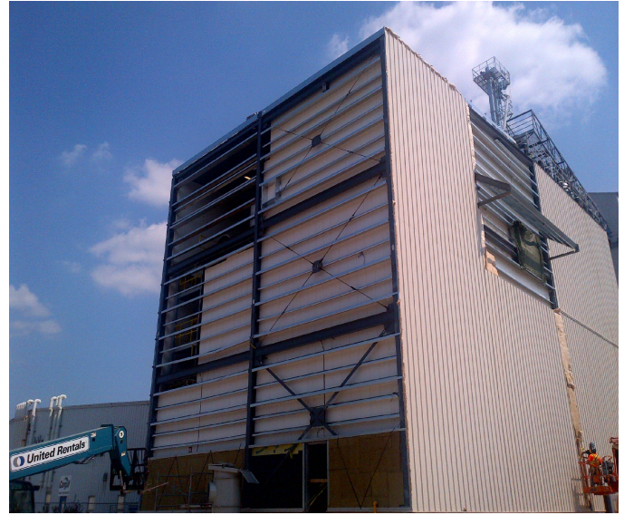
Enclosing 14 new storage bins and extrusion process tower at Agribrands’ animal feed manufacturing facility expansion in Strathroy, Ontario.
