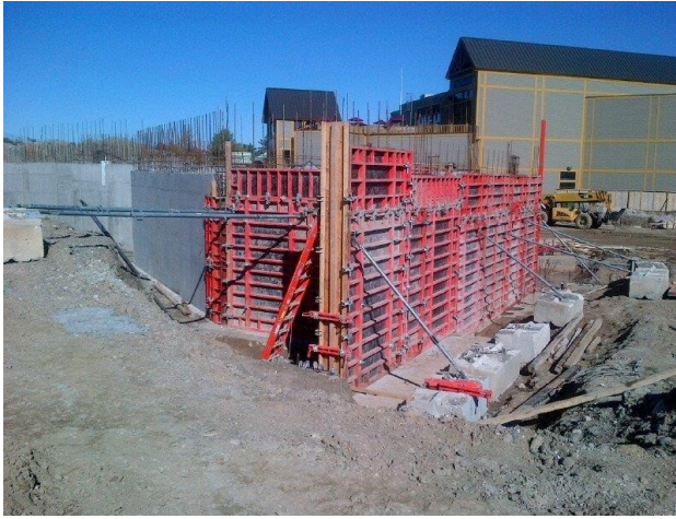
Concrete foundations being poured for the new convention centre at Blue Mountain Resorts.
