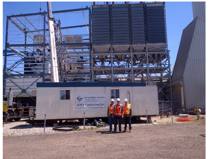
Agribrands' plant expansion underway. L to R: KMA's Chris Dewsbury, Robert Box and Keith McEwen.
