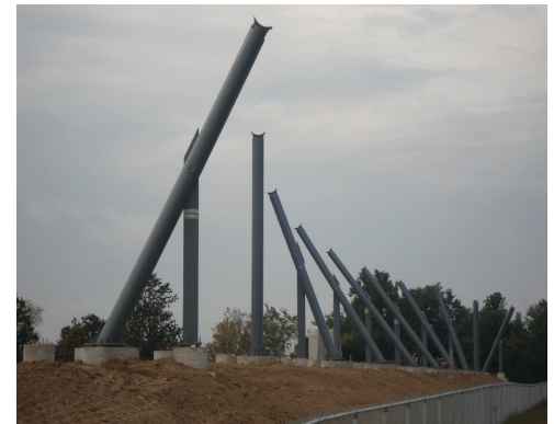
In less than 12 weeks 136 tons of epoxy coated architectural steel was fabricated and installed.
