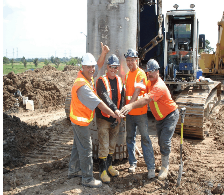
John Belsito (left), KMA Field Superintendent, teams up with the Deep Foundations crew to install (22) 1-meter diameter caissons.
