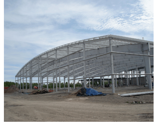
Structural steel over rinks 3 and 4
