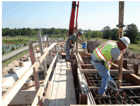
The foundations for the structural steel frame required the construction of 600 lineal feet of grade beams, including the supply and placing of approximately 36 tons of rebar and over 400 cubic meters of concrete.
