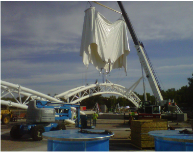
Cover for the performance stage being lifted into place. Arch supports ready for connection.
